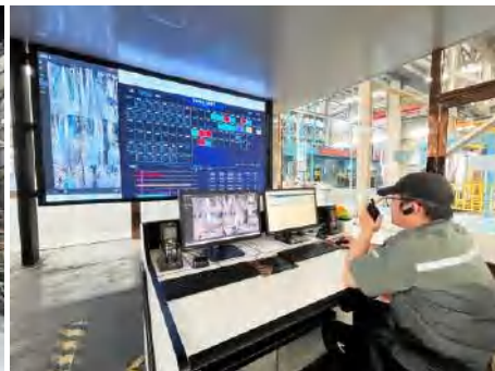
Central Control Room
